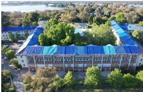
Figure 3: hail damage to Univeristy House in 2020
